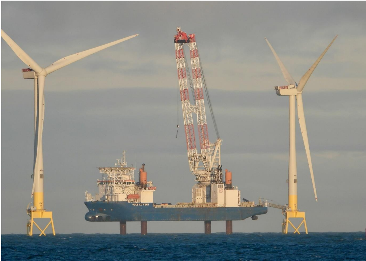
Plate 5.8 Example jack-up vessel used for WTG installation - Vole au vent (Morecambe Offshore Windfarm Ltd, 2023)
